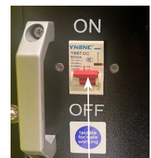
Switch in 'on' position
